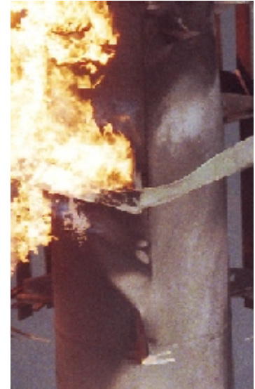
Visible Crack in Flare Body
